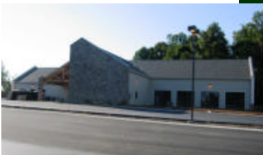
A view from the parking lot as the Exeter Library enters the final stage of construction.
